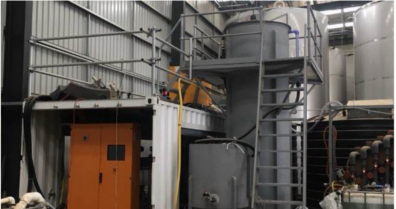
Commercial Plant to Remove PFAS from Leachate
